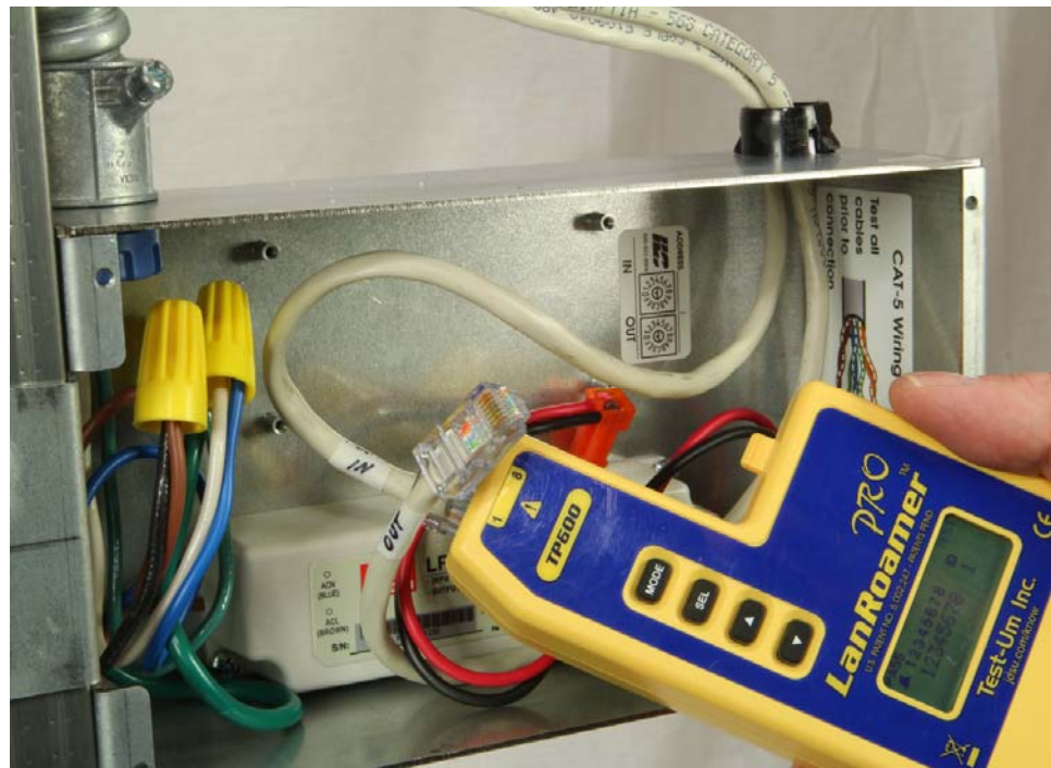
Figure 5 Testing Data Line
